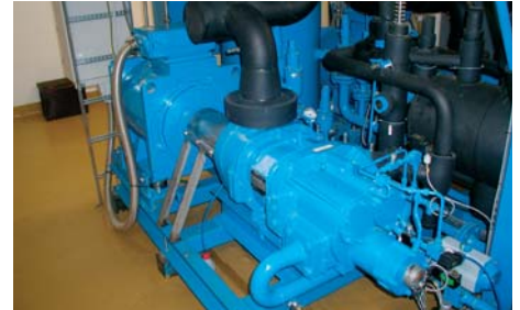
Ethyleneglycol Chiller Unit
